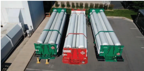
Figure 1. Compressed hydrogen stored in tanks as a fuel for back-up fuel cells in Microsoft Salt Lake City data center [8]
