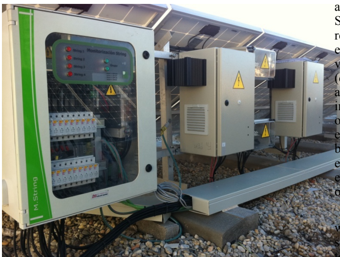
Fig. 8. Green Power Technologies solar inverter system
